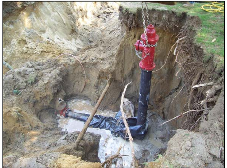
A new hydrant being installed in South Burlington by the CWD Retail Department
