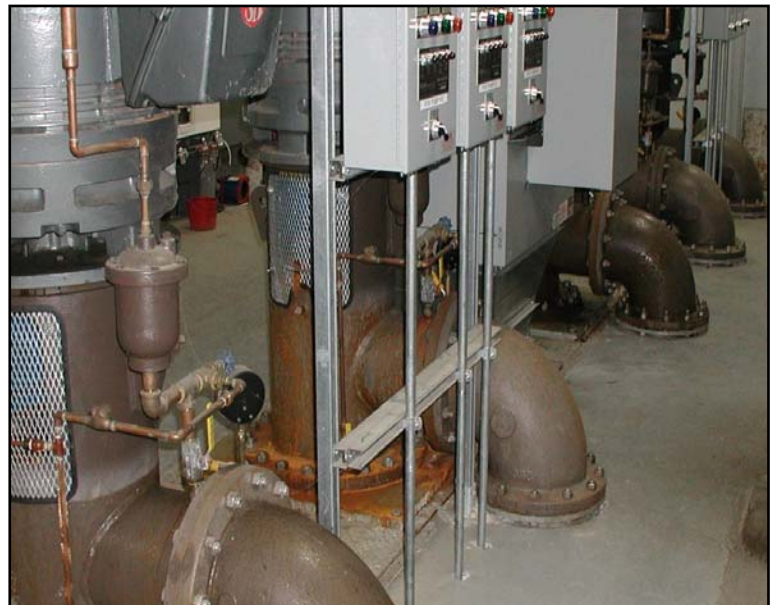
Raw Water Discharge Piping
